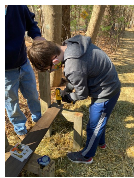
Fellow scout Darwin Block putting the finishing touches on the benches at the farm.
